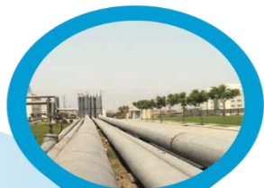
Heating pipe network
